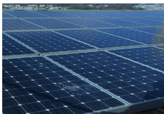
Solar PV modules installed on the Guildhall
